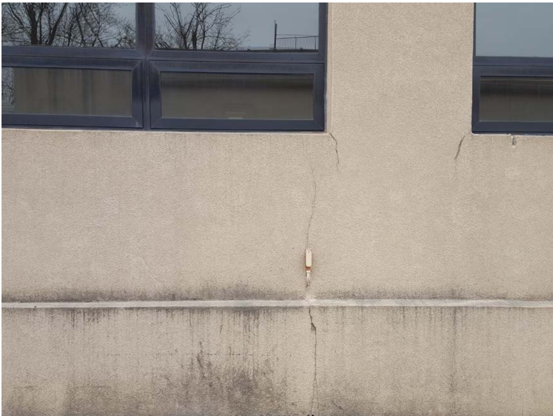
Photo #8 – Stress Cracking in Exterior Wall (North).
