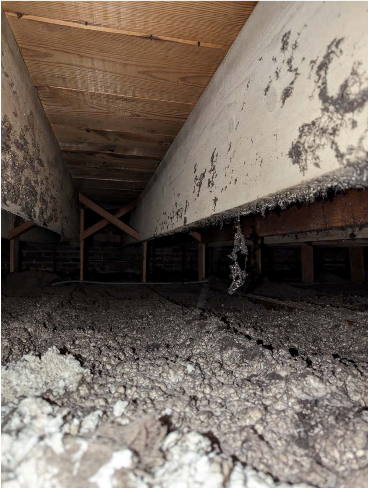
Photo #15 – View of Ceiling Cavity below Roof at Non-water Damaged West End.
