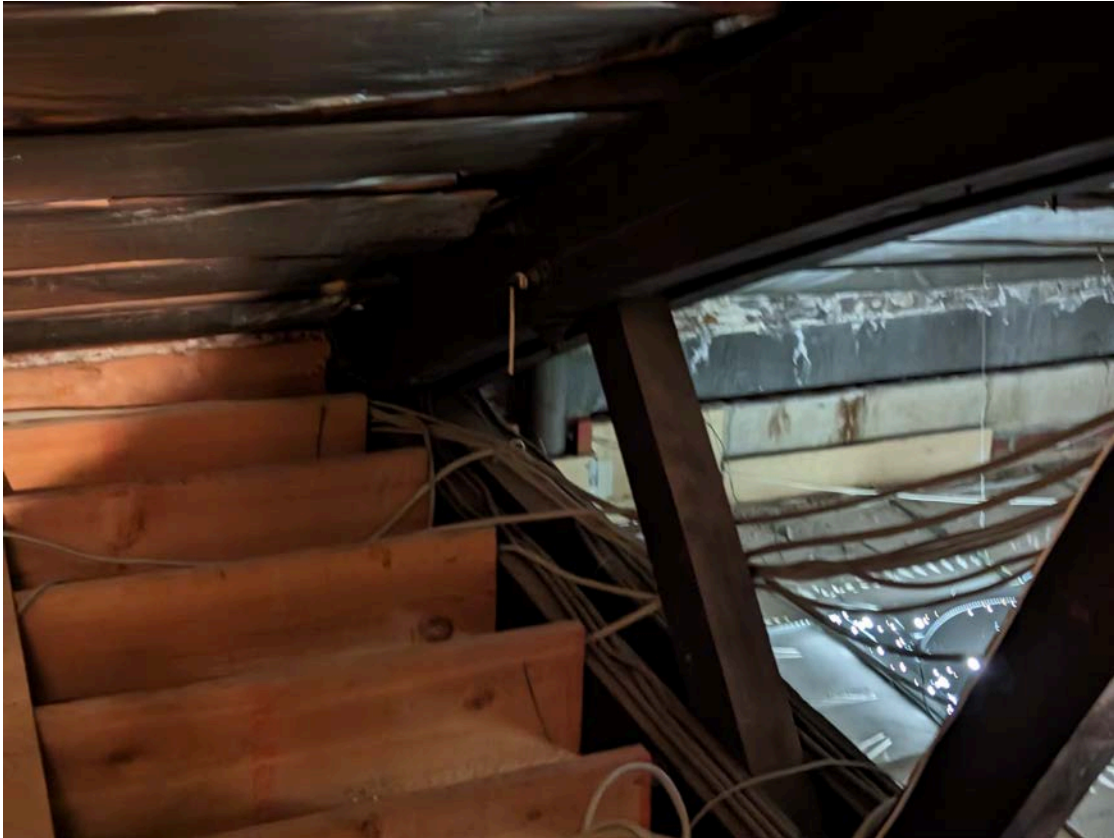
Photo #19 – 2x Ceiling Joists without Hangers to Truss.
