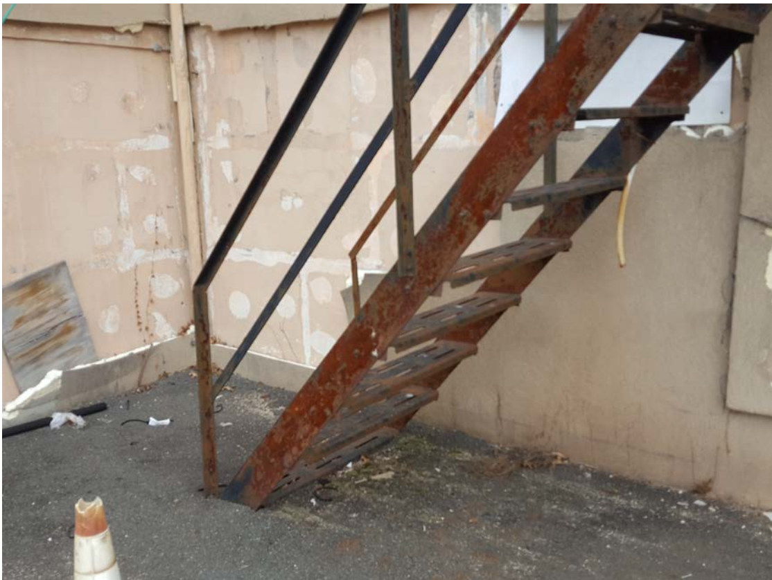
Photo #10 – Surface Rusted Fire Escape & Large Sections of EIFS Removed/Missing.
