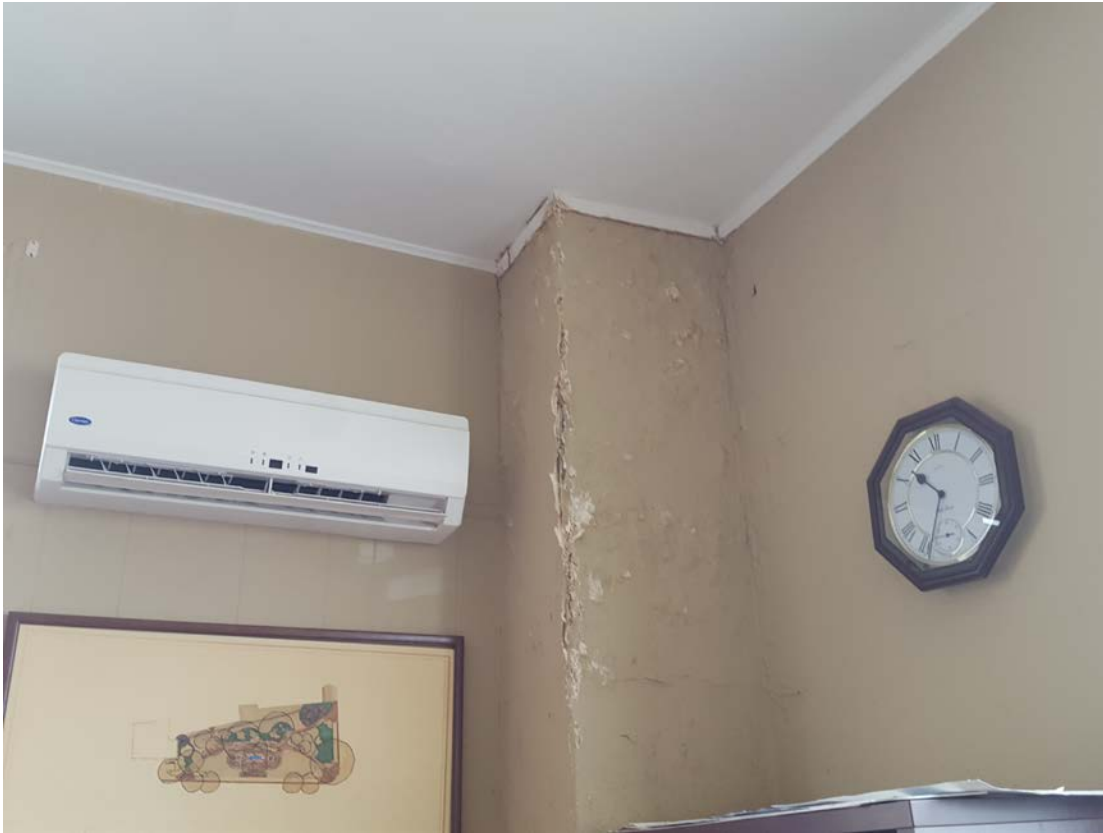
Photo #13 – Southwest Corner Chimney/Chase with Water Damage.
