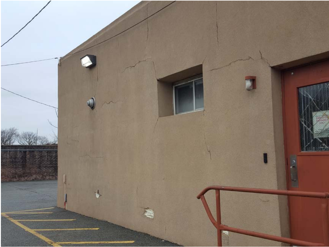
Photo #9 – Stress Cracking in Exterior Wall (East).
