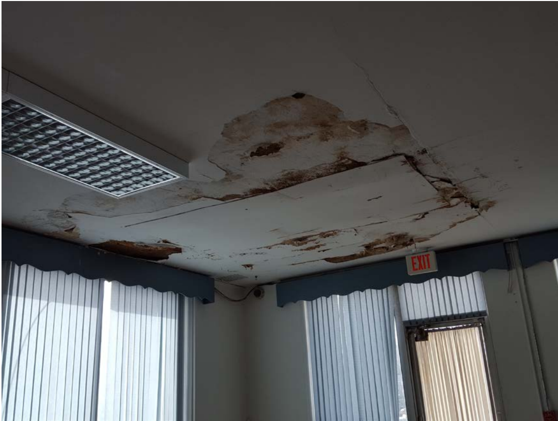
Photo #11 – Water Damaged Ceiling at Southeast End of Courtroom.
