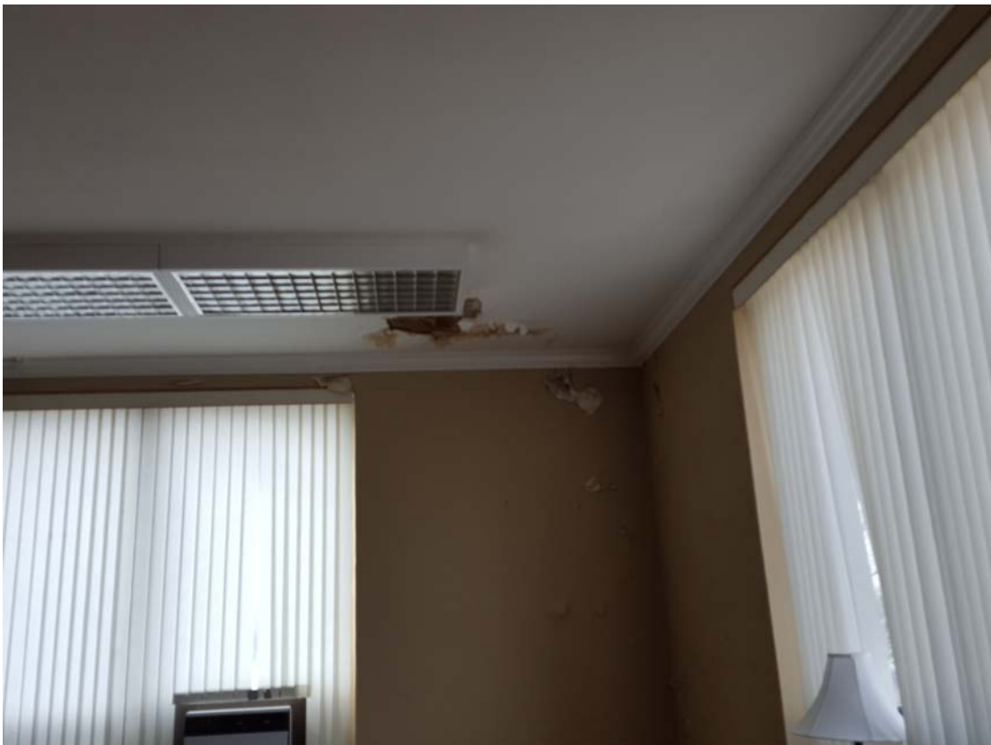
Photo #12 – Water Damaged Ceiling Northwest Corner.
