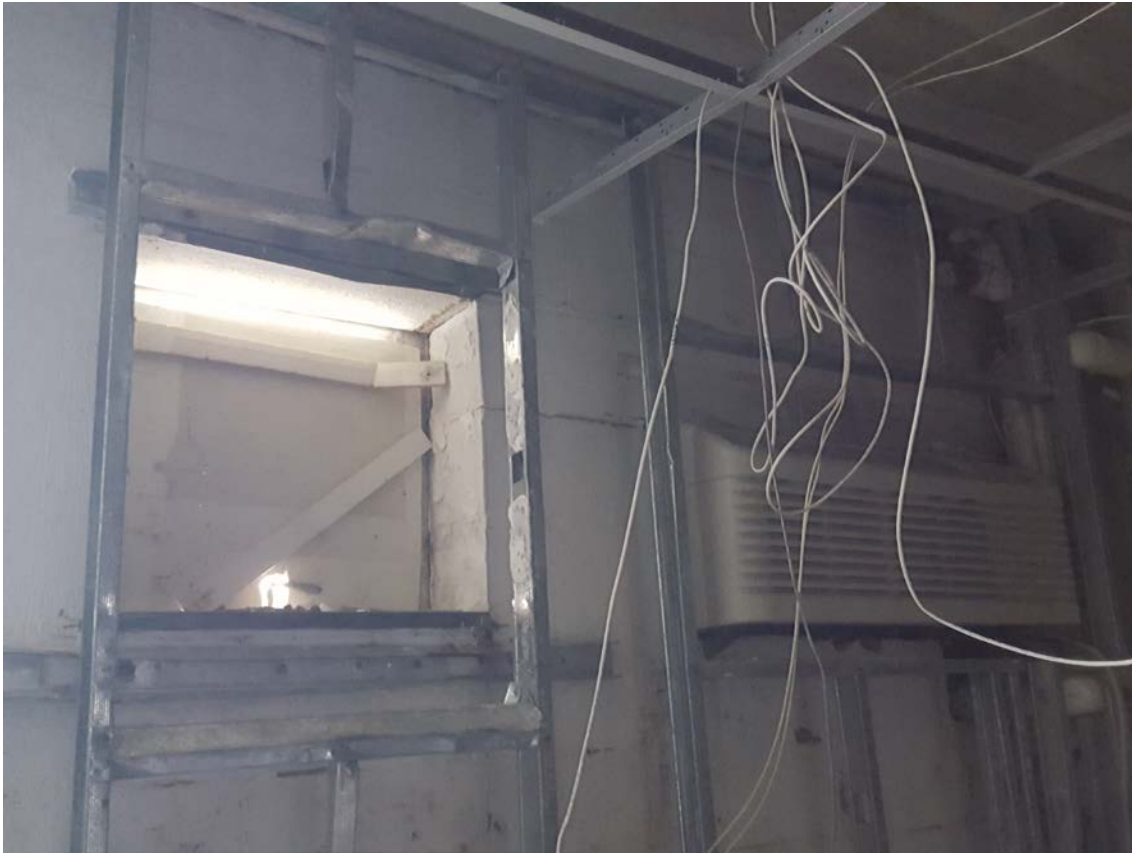
Photo #31 – Horizontal Cracking Between Basement Openings – East Side.
