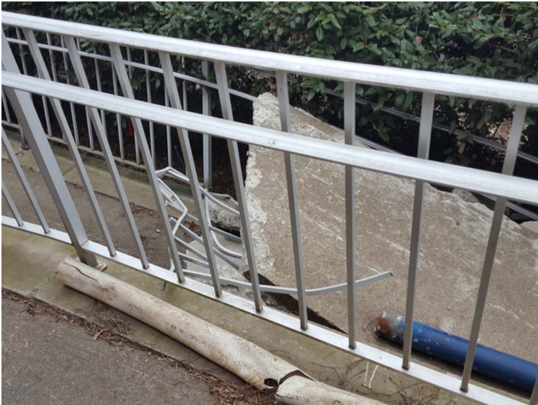
Photo #12 – Damaged Front Entry Ramp.
