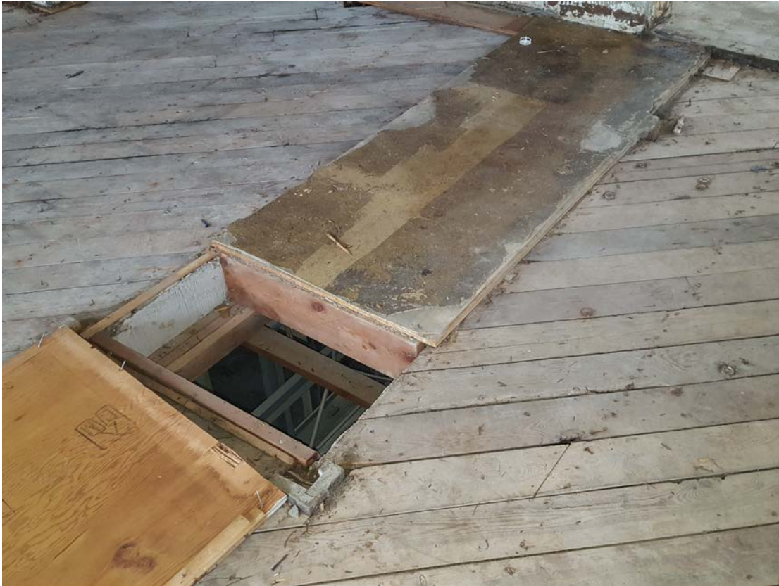
Photo #17 – Opening in Floor with Miscellaneous Blocking & Loose Plywood Covering.
