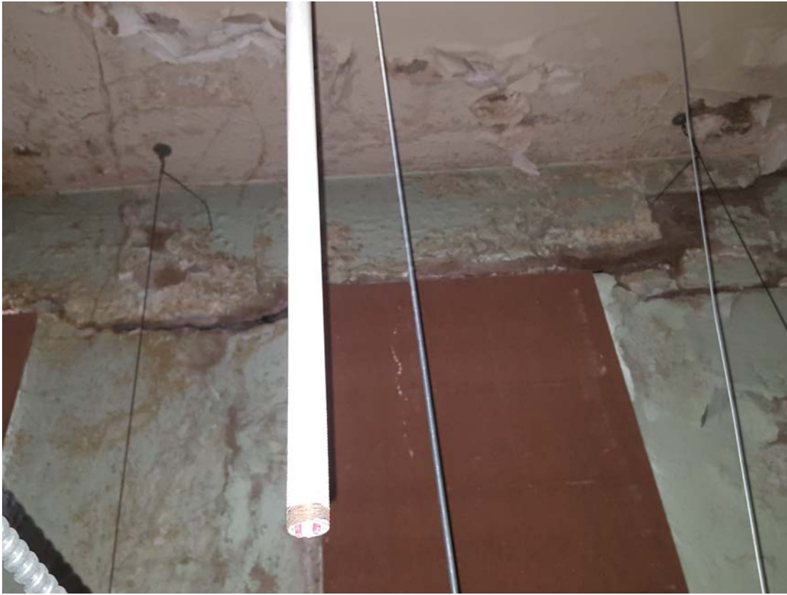
Photo #23 – Horizontal Masonry Cracking at Southwest Section – Located at West Wall.
