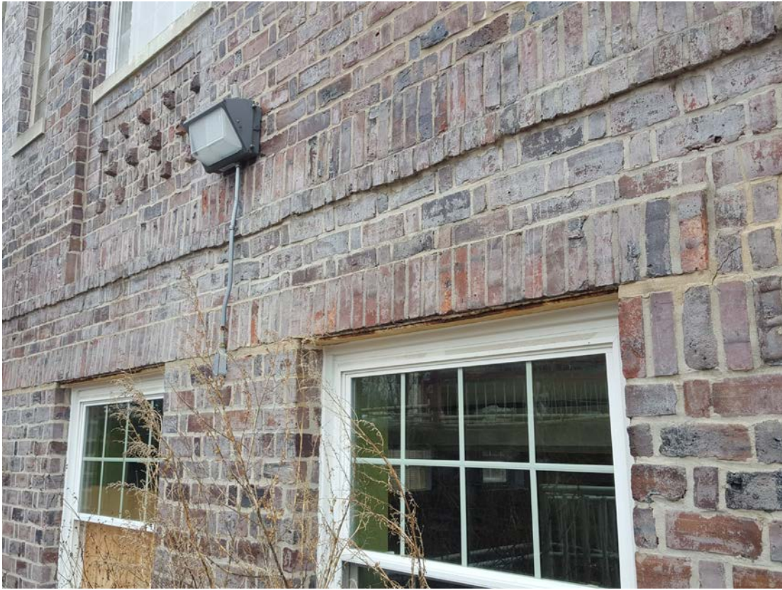
Photo #9 – Deteriorated Steel Lintels over Windows.
