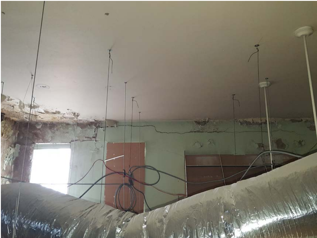
Photo #22 – Horizontal Masonry Cracking at Southwest Section – Located at South Wall.
