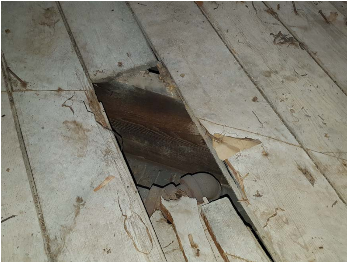
Photo #16 – Damaged Floor Sheathing Sporadic Throughout Wood First Floor.
