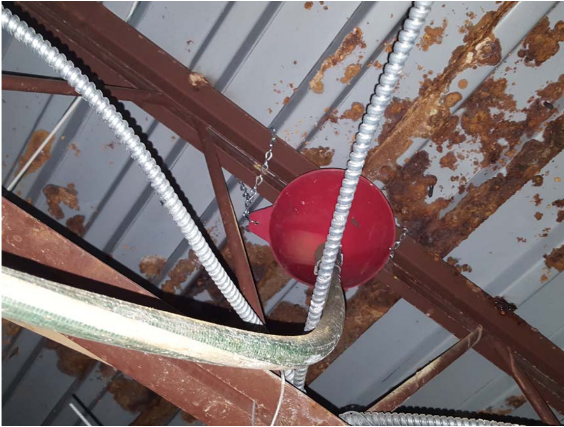
Photo #25 – Deteriorated Metal Roof Deck Plus Makeshift Drain & Hose.
