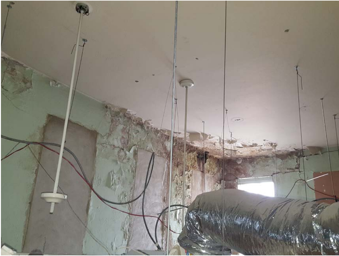
Photo #21 – High Moisture Damage above Photo #20.
