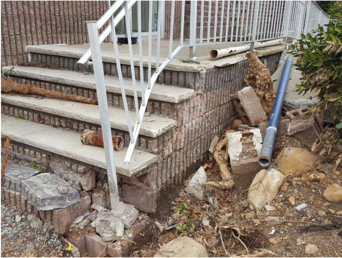
Photo #11 – Damaged Front Entry Steps, Guardrail & Ramp.
