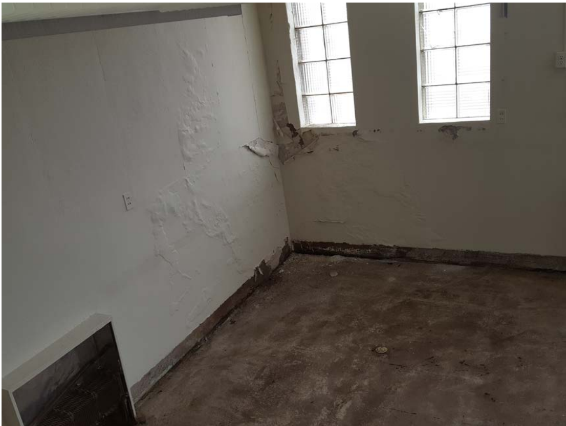
Photo #20 – Moisture Damage of Interior Finish/Paint Located at Southwest Section.
